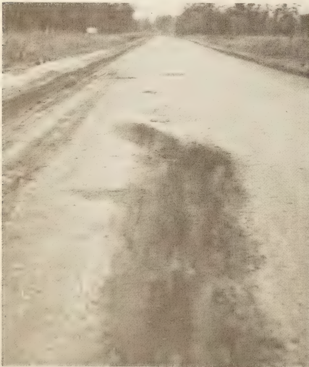
FIGURE 13.—POOR DRAINAGE RESULTED IN THE UNSATISFACTORY CONDITION OF THIS AREA OF EXPERIMENT 3 NEAR STATION 363. ANALYSES OF MAT AND SUBGRADE FROM THIS AREA ARE GIVEN IN TABLE 7.
